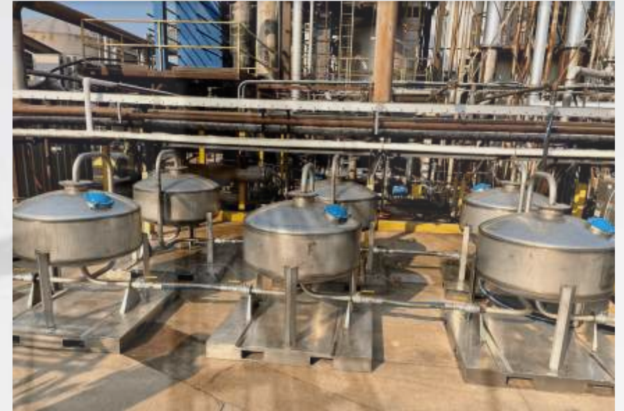
PE3 Pods for dosing and mixing ionic fluid into oil
